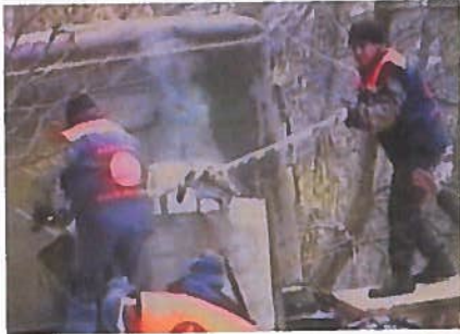
DANGER Crews recover radioactive containers in former Soviet Republic of Georgia.
